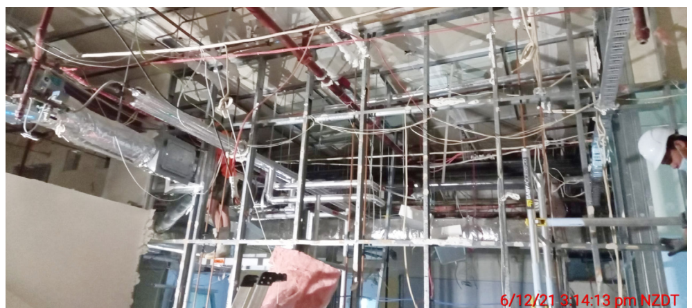
The creation of a new Day of Surgery Admissions and Recovery Area is well underway. Much of the work for this project is behind the walls, under the floor and above the ceiling to get the electrical, air conditioning, heating, ventilation, fire and medical gas systems in place.
