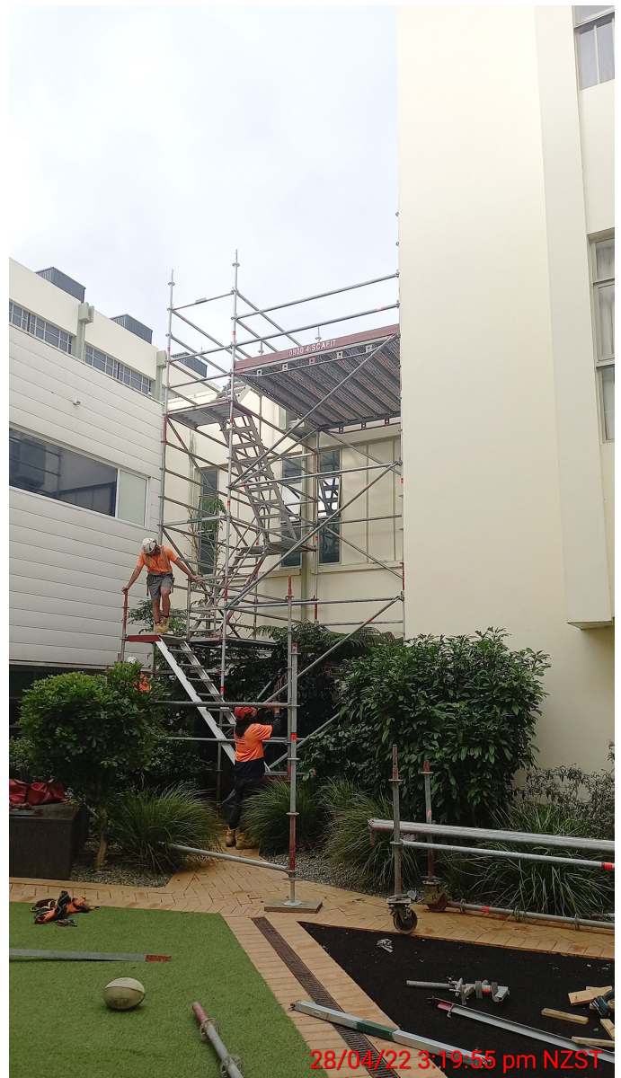
Access to the roof installed so the roof-top plant room can be built.
