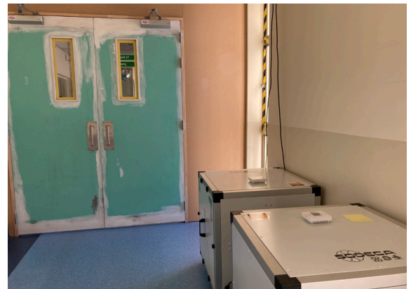
Two sets of doors established in the corridor, with high volume air scrubber placed in area, to assist air control.
