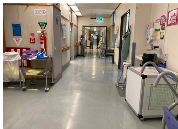
High volume scrubbers throughout ward.
