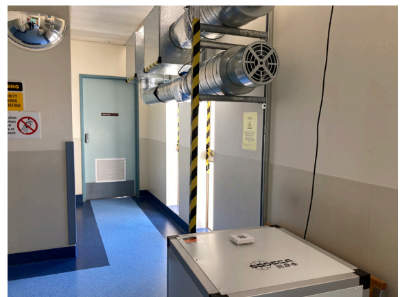
Suction unit in corridor, together with high volume air scrubber, creates negative pressure zone.
