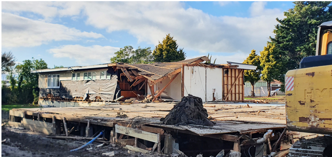
Final stages of the disassembly of Pullar Cottage, making way for the new Acute Mental Health Unit.
