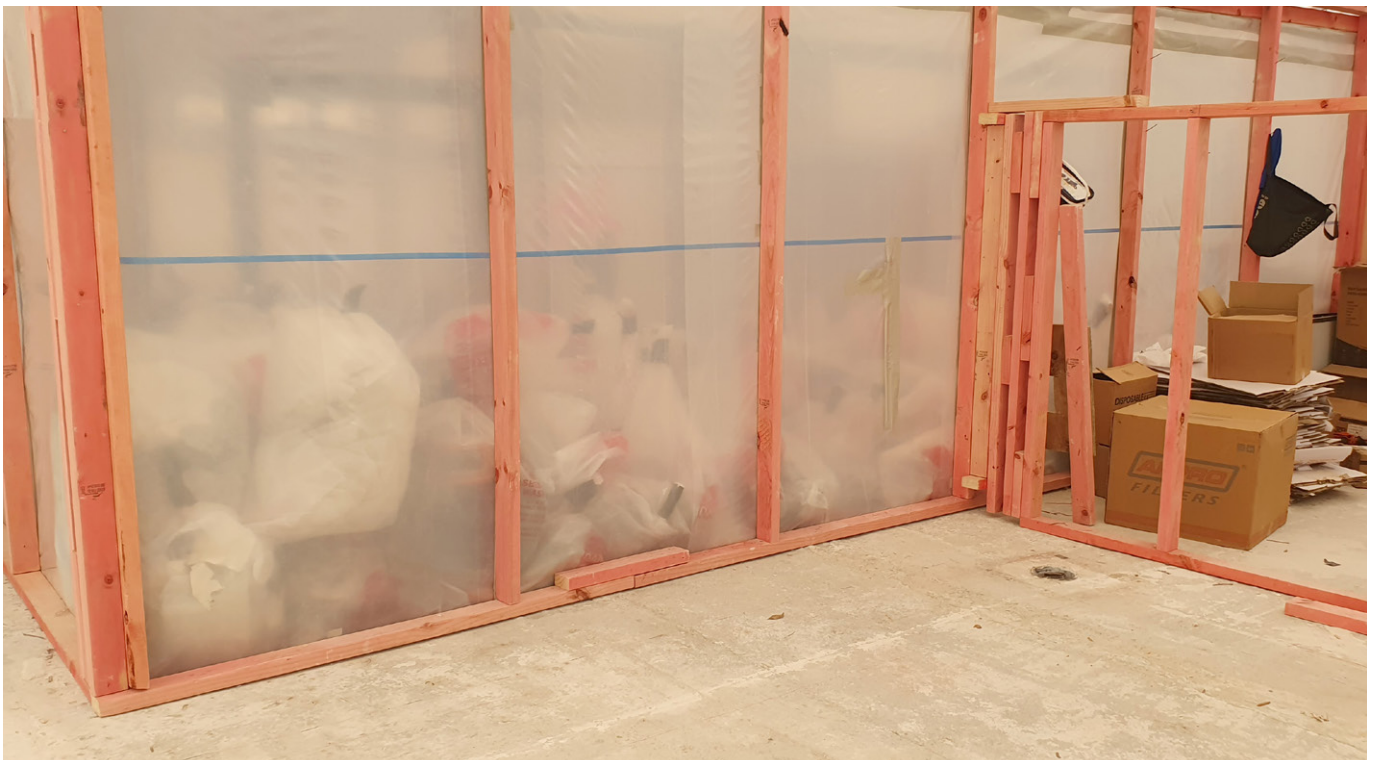
Waste material removed is double-bagged and stored in secure compartment awaiting planned removal off site
